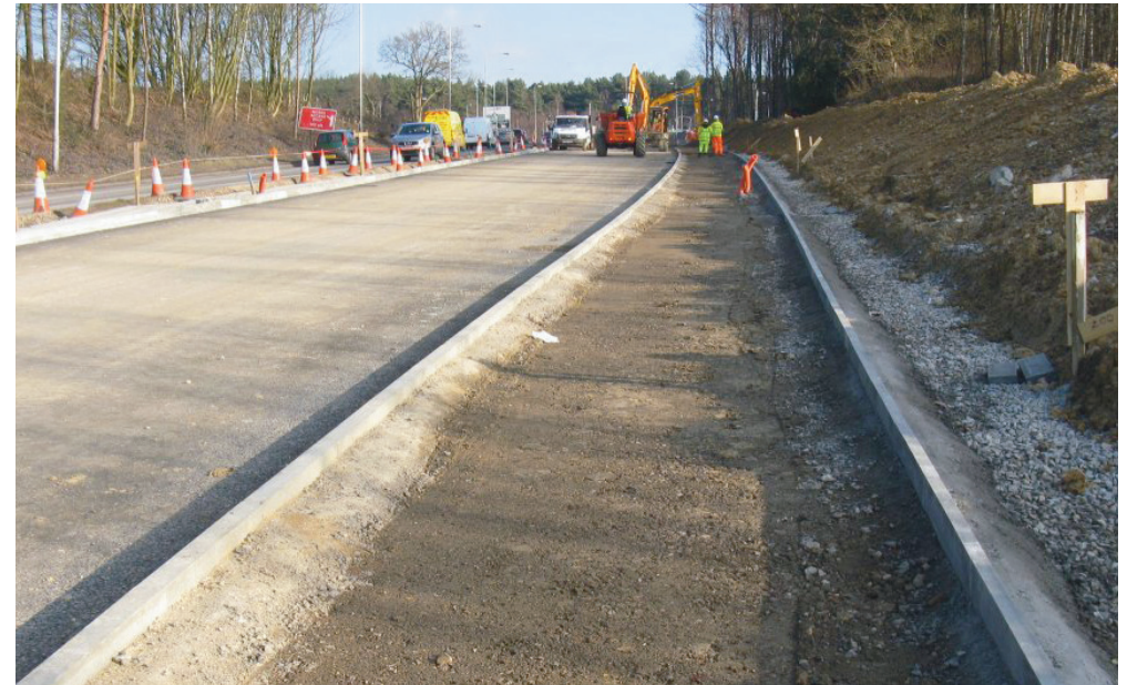
Construction work for North Farm Improvements (Tunbridge Wells), part-funded by the Department for Transport's Local Pinch Point Fund
